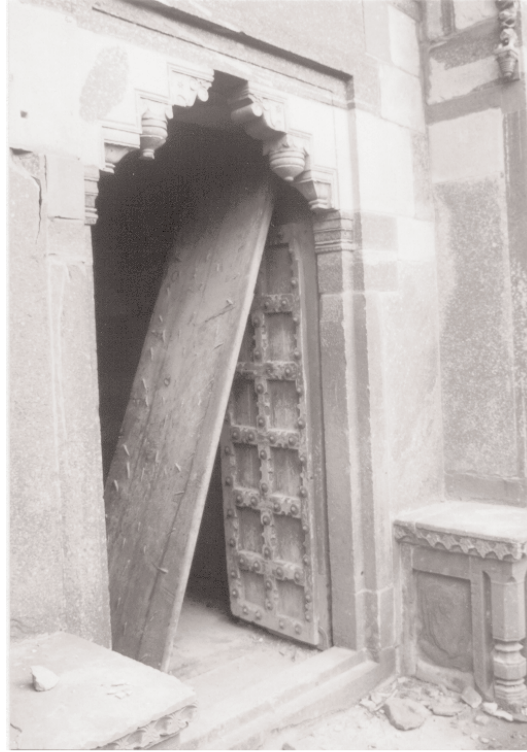
Fig. 4 Rang Mahal: In need of preservation.
